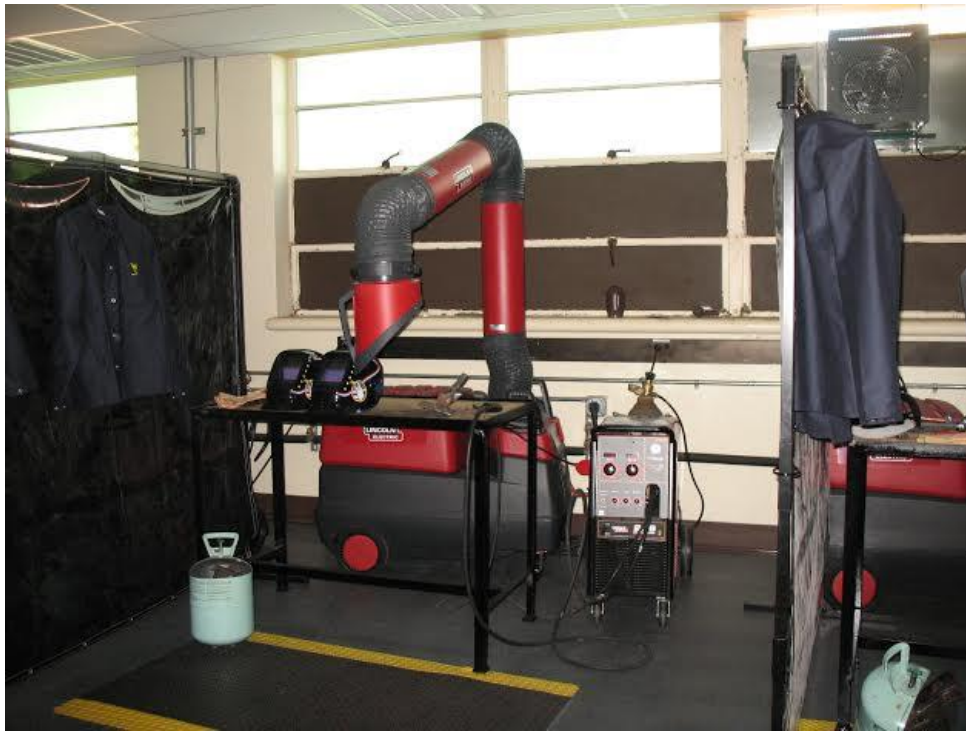
Figure 1.7 Mechanical Engineering Fusion Welding Laboratory
